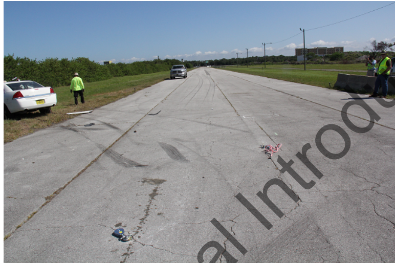
Figure 6.1: Roadway Evidence Photos
